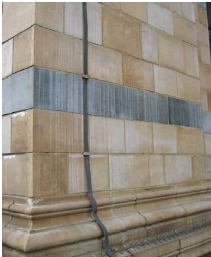
4 Terracotta blocks etched by poorly controlled acid cleaning, leaving the substrate vulnerable to further decay
