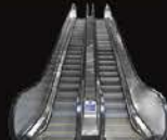
Escalators and moving walkways
